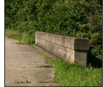
Detail of Hoffman Creek bridge at US 51. The bridge is listed on the National Register
